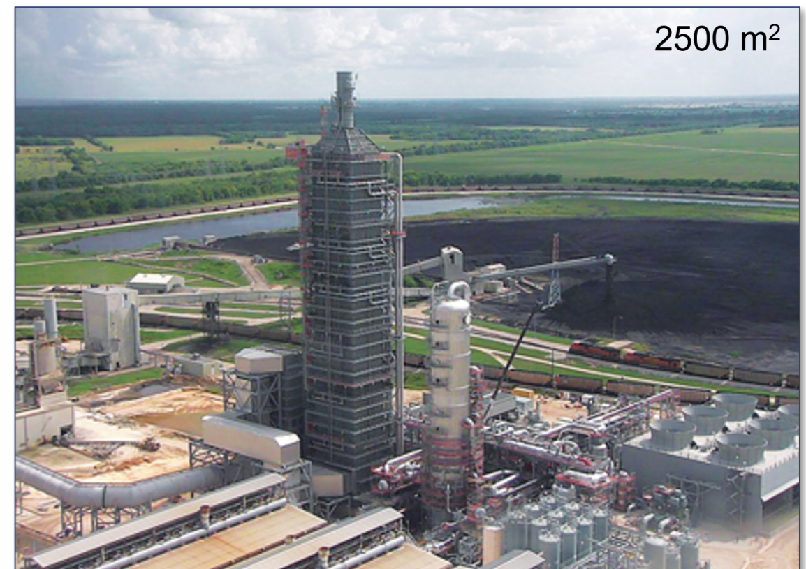
PETRA NOVA ABSORBER TOWER Thompsons, TX
